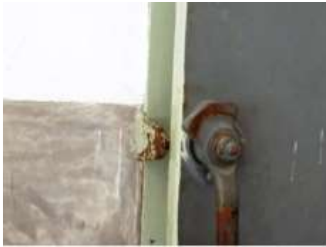
Photo 9: Exit door obstruction.
